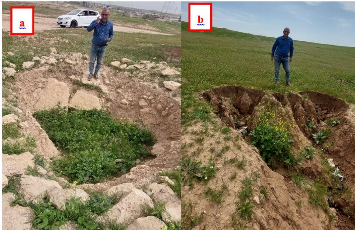
Fig. 18. a: karst in Al Athba Valley due to gypsum dissolution and collapse of marle and limestone above it; b: neck point phenomena in the soil of Al Athba Valley.
